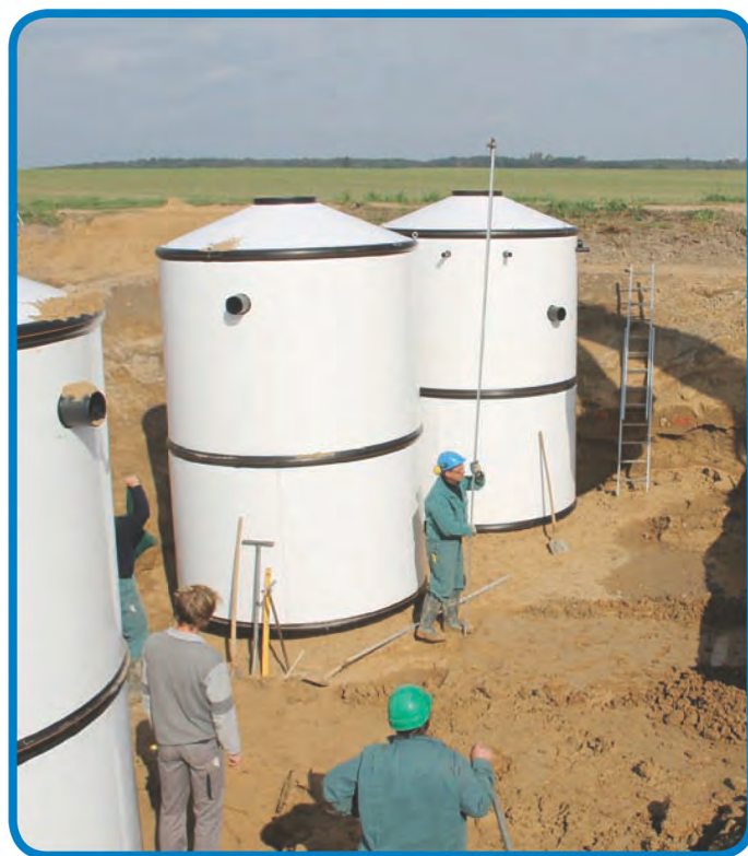
Installation of a 220 PE wastewater treatment plant for the village of Remlin near Rostock, Germany, in October 2011
